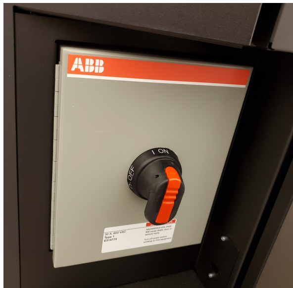
Figure 154: Electrical disconnect switch in ON position
