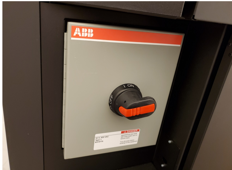
Figure 159: Electrical Disconnect OFF
