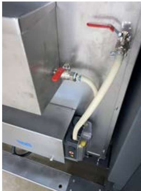
Figure 204: Vat and reservoir valves (closed position)
