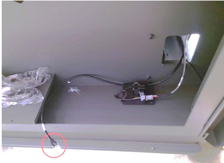
Figure 28: Cat 5e communication cable
