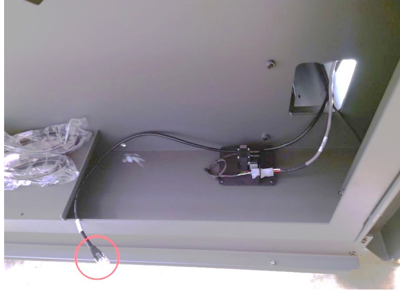
Figure 28: Câble de communication Cat 5e
